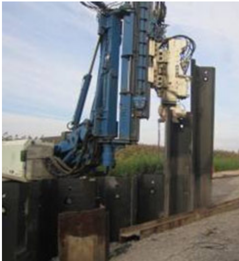
Each panel is installed by a vibratory hammer and driven to a depth of up to 77 feet.
