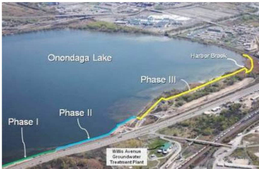
Steel work for the nearly 1 ½ mile underground barrier wall is now complete.
