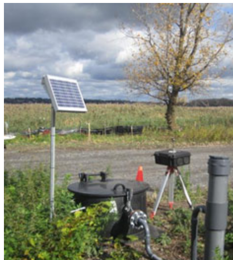
Solar-powered monitoring system.
