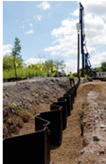
A GPS unit is used to confirm panel alignment. The barrier wall includes 1,620 panels.
